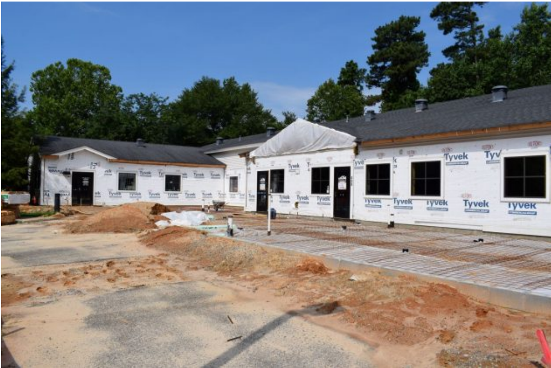
Updates to Heritage Humane Society's Expansion Project as of July 6, 2021 (Courtesy of Heritage Humane Society)
