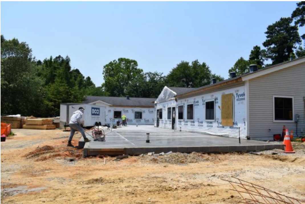
Updates to Heritage Humane Society's Expansion Project as of July 6, 2021 (Courtesy of Heritage Humane Society)
