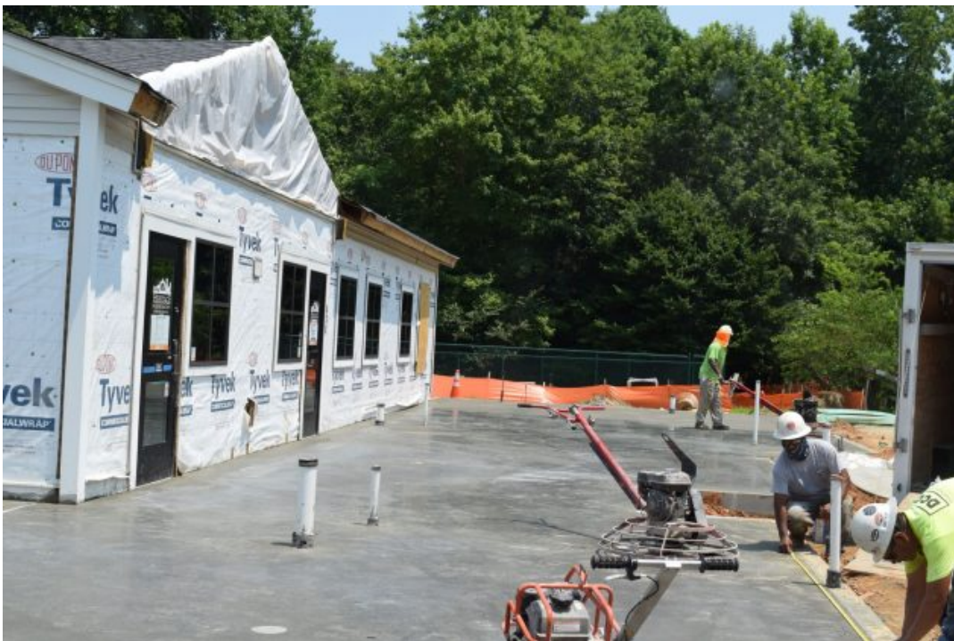
Updates to Heritage Humane Society's Expansion Project as of July 6, 2021 (Courtesy of Heritage Humane Society)
