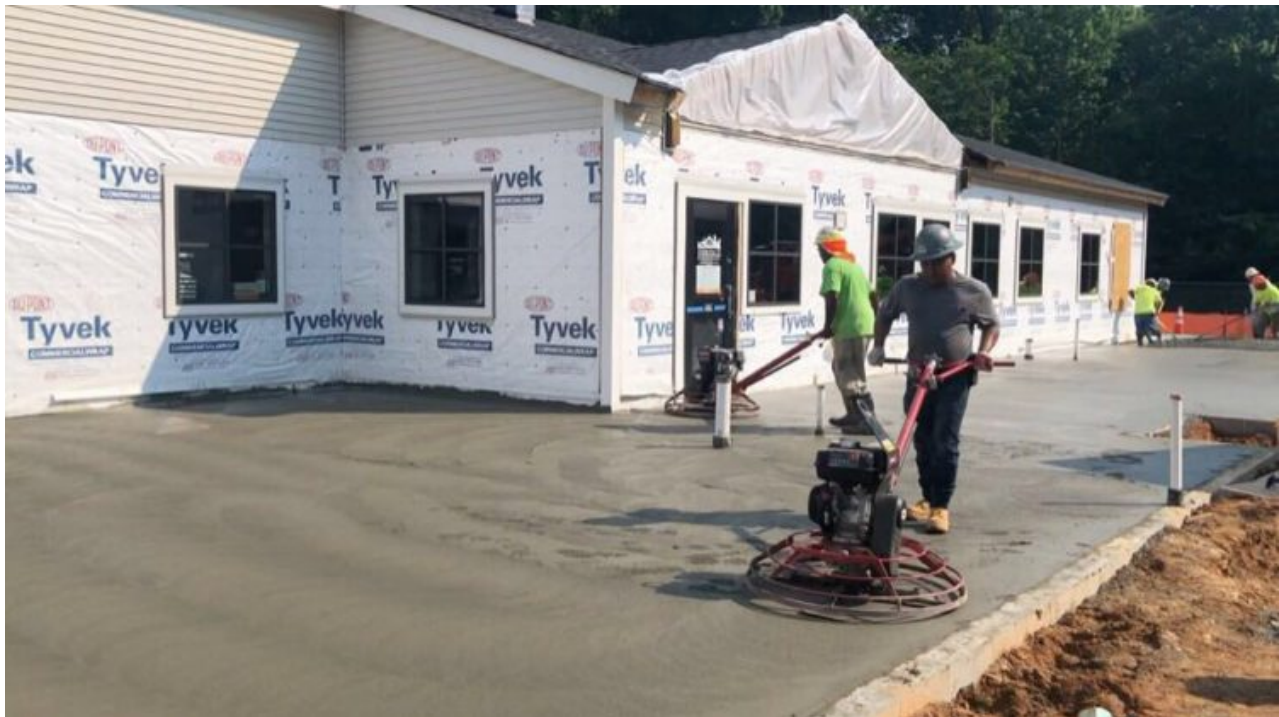
Updates to Heritage Humane Society's Expansion Project as of July 6, 2021 (Courtesy of Heritage Humane Society)
